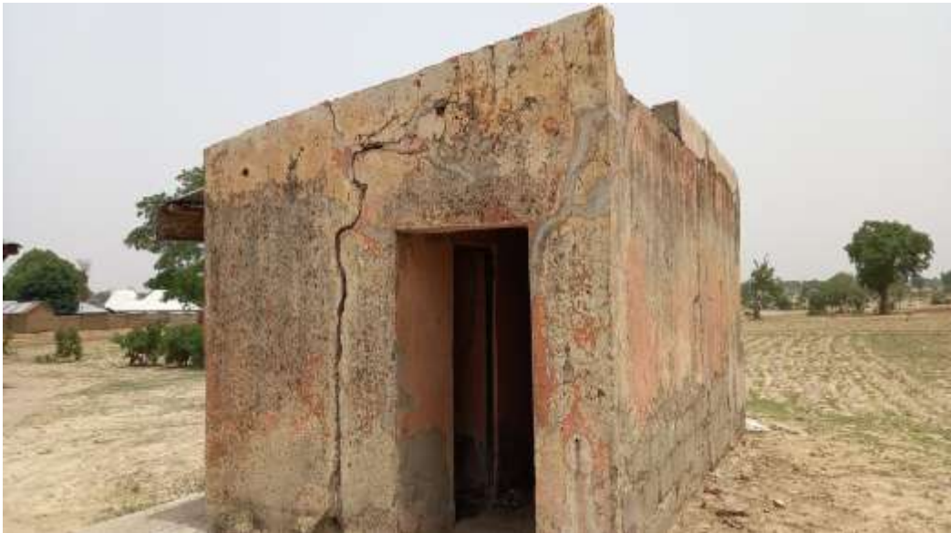
B Dilapidated lavatory built by MVP
